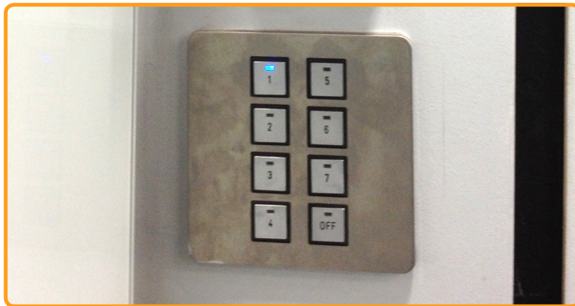
above: example of unlabelled lighting control
