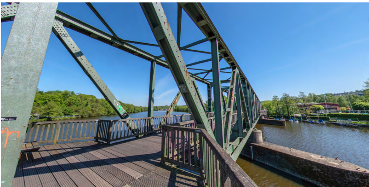
Figure 7. The Eisenbahnbrücke Kupferdreh is a former railroad bridge that crosses the River Ruhr in south-eastern Essen, today a cycling and hiking path. | Google Street View, 2023.
