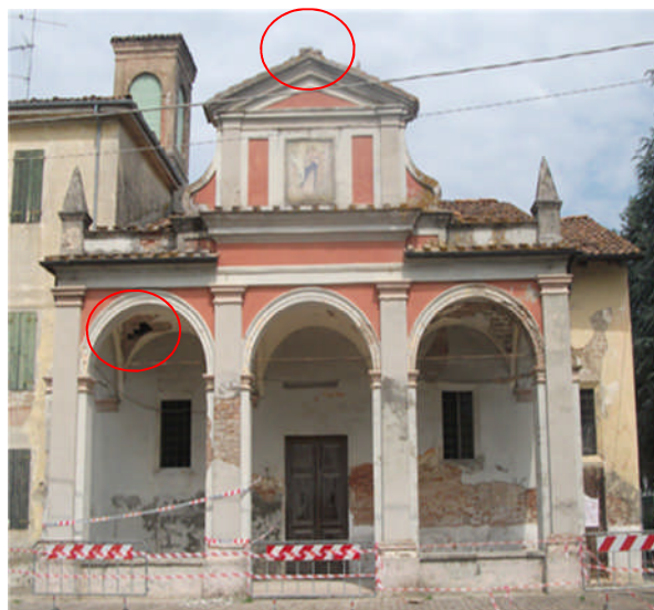
Figure 4.30. – Slightly damaged façade of the Oratorio in Corpo Reno.
