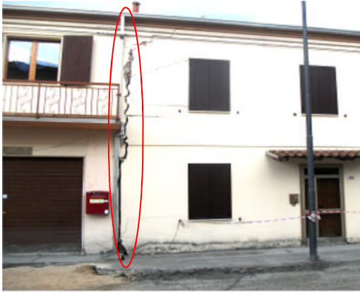
Figure 4.8 - Large and extensive vertical cracks on a residential house near the church of S. Pavlo in Mirabello.
