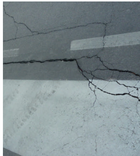
Figure 3.7 - Detail of lateral spreading in the street of Mirabello.
