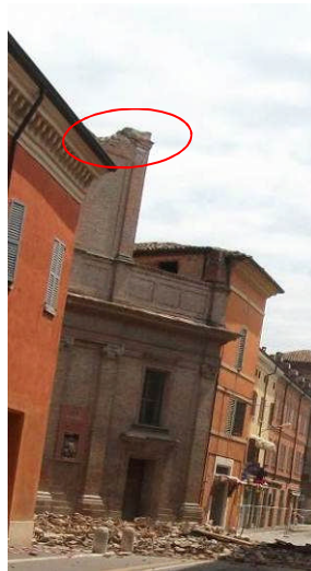
Figure 4.25 - Collapse of the top end of the facade of the Duomo in Finale Emilia.
