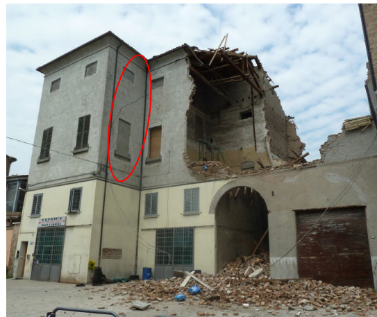
Figure 4.18. - Partial collapse of a commercial building in via Cesare Frassoni in Finale Emilia.
