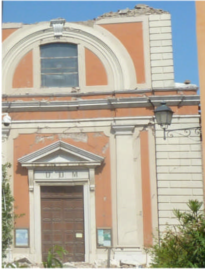
Figure 4.27 - Partial collapse of the façade of the church of D.O.M. in San Felice sul Panaro.
