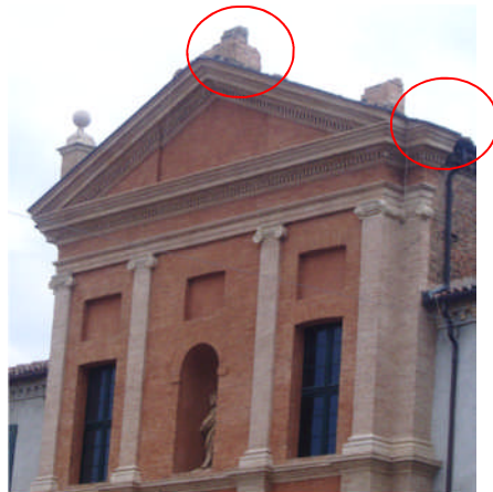
Figure 4.19 - Dislodged decorations of the façade in the church of S. Bartholomew in Finale Emilia.
