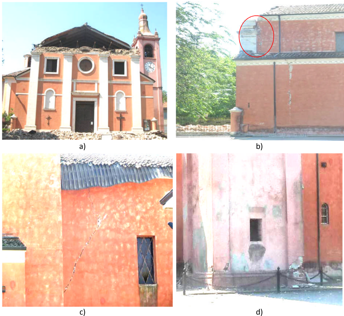
Figure 4.24 - Church on via degli Estensi in San Felice sul Panaro: a) Collapse of the top façade of the church on via degli Estensi; b) Cracks on the external wall of the façade and the south wall of the church on via degli Estensi; c) Large and extensive crack on the north side of the church on via degli Estensi; d) Spalling at the bottom of the bell tower of the church on via degli Estensi.
