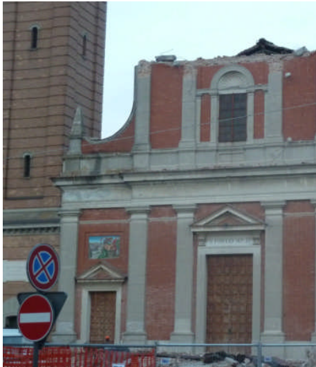
Figure 3.4 - Damage to facade of the Church of Mirabello (front view).
