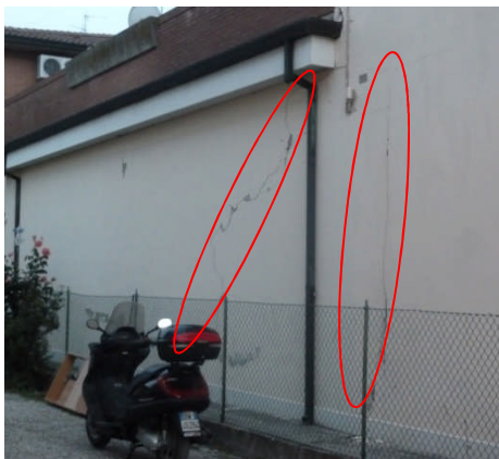
Figure 4.10 - Long cracks on a residential house near the church of S. Pavlo.
