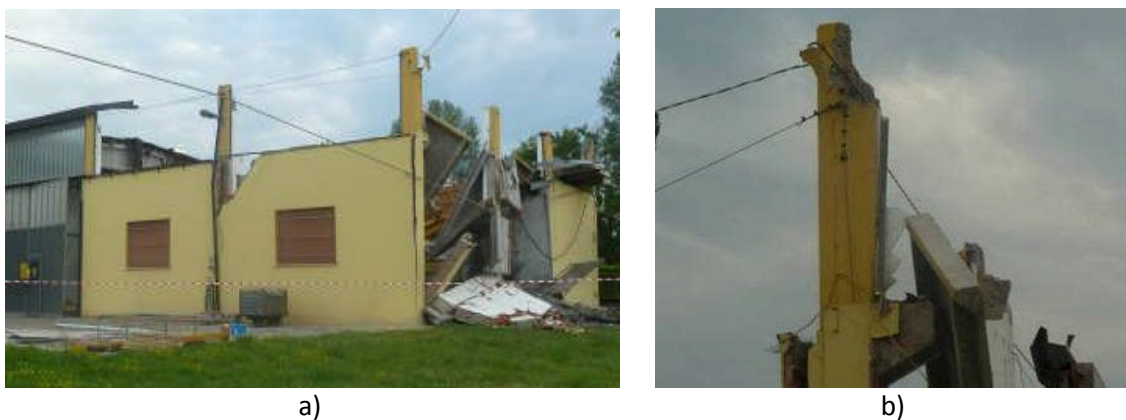
Figure 4.38 - Industrial buildings close to Mirabello: a) overview of the pre-cast structure; b) joint detail.
