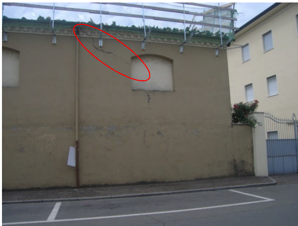
Figure 4.17. – Dislodged ceramic tiles from the roof and Shear crack on the wall of a residential building in Finale Emilia.
