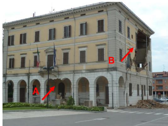
Figure 3.11 - Damage to the town hall of S. Agostino. Detail A – Fallen column. Detail B – Collapse of the external wall.
