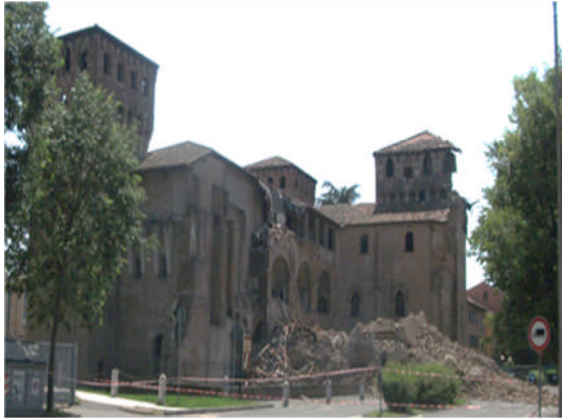
Figure 4.34 - Partial collapse of the east side of the Castello delle Rocche in Finale Emilia.
