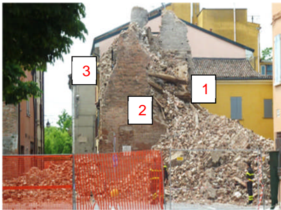
Figure 4.33 - Collapse of a brick masonry clock tower in piazza Alfredo Baccarini in Finale Emilia.
