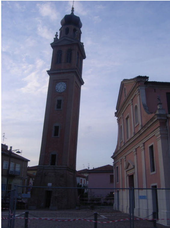
Figure 3.2 - Damage to the Church of Nativita' di Maria and Clock tower in Vigarano Mainarda
