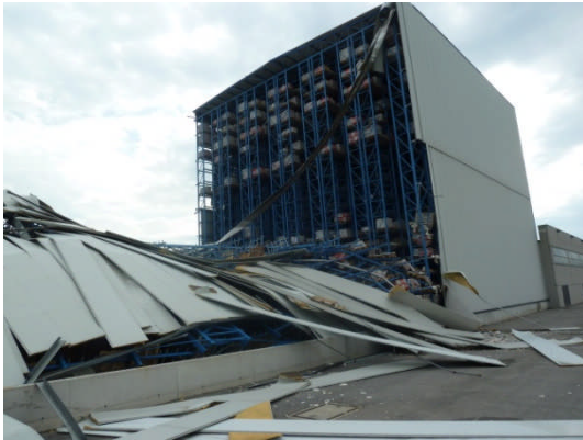
Figure 3.11 - S. Agostino Ceramic – Collapse of a warehouse for the storage of ceramic tiles.
