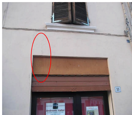
Figure 4.6 - Light damage of a commercial/residential building adjacent to the church of Nativita di Maria.
