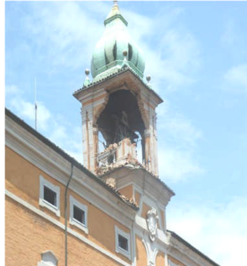
Figure 4.32 - Collapse of a column supporting the bell on a clock tower in Finale Emilia.
