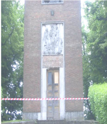
Figure 4.31 - Dislodged decorative marble plates from the brick masonry tower in Finale Emilia.
