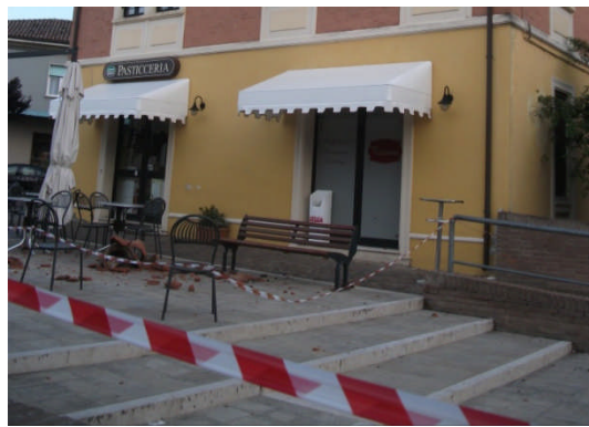
Figure 4.5 - Dislodged chimney of a commercial/residential building in Vigarano Mainardo.
