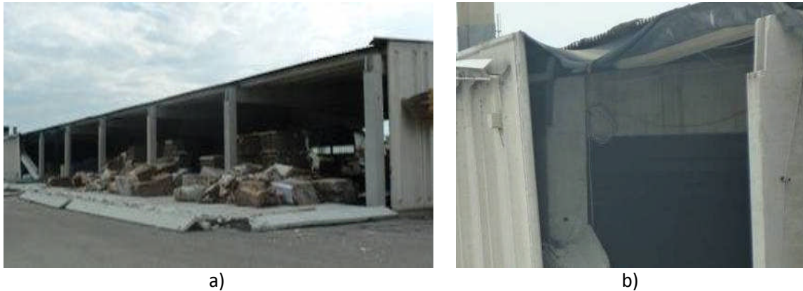
Figure 4.43 - Industrial building close to Sant Agostino: a) overview; b) panel connection failed.
