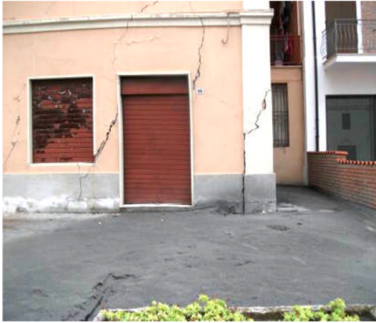
Figure 4.12 - Large and extensive cracks due to differential settlement on a residential house in San Carlo.
