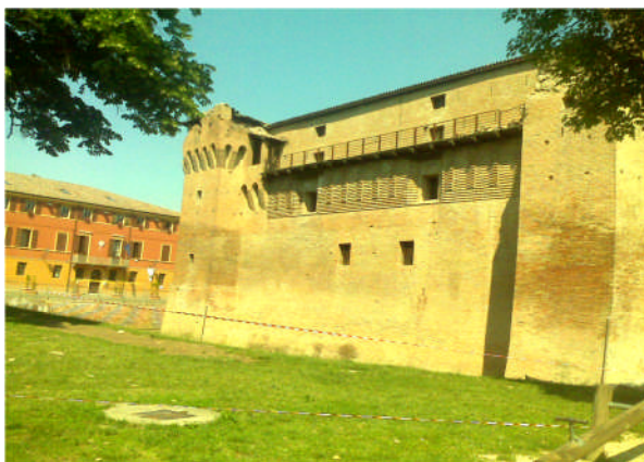
Figure 4.36 - Partial collapse of the fourth tower of the Rocca Estense Castle.
