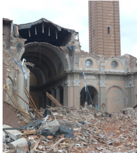
Figure 3.5 - Damage to cupola of the church of Mirabello (back view).
