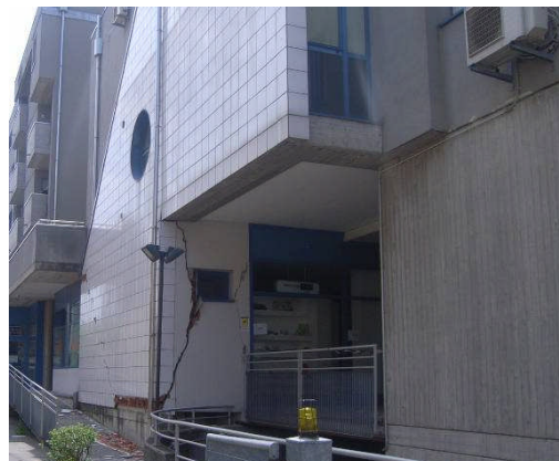
Figure 4.3 Residential building in Finale Emilia with damage in the hollow clay brick infill.
