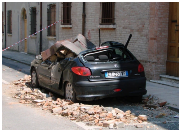
Figure 7.1 - Car crushed by falling chimney, Finale Emilia.
