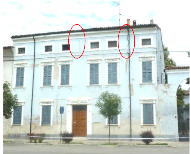
Figure 4.16 - Cracks on the wall of the 3 rd floor in a residential building via Cesare Frassoni.
