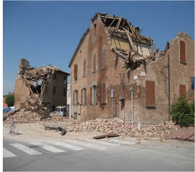
Figure 4.28 - Partial collapse of the church buildings next to the church of D.O.M.
