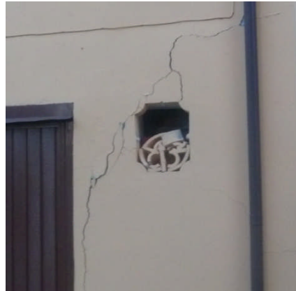
Figure 4.9 - Long crack on a residential house near the church of S. Pavlo.
