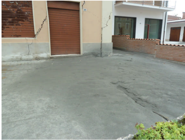
Figure 3.8 - Damage to a residential building in S. Carlo. The picture shows clear evidences of liquefaction.
