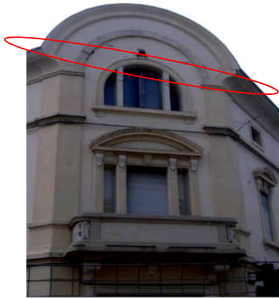
Figure 4.15 - Light damage of a commercial/residential building in piazza Giuseppe Garibaldi in Finale Emilia.
