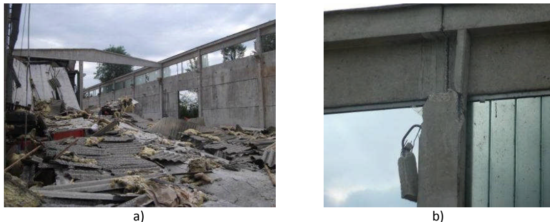
Figure 4.52 - Industrial building in Sant Agostino: a) overview; b) joint failed detail.
