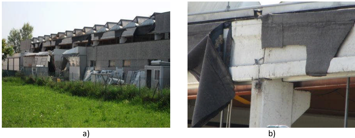
Figure 4.56 - a) Warehouse structure with H-section longitudinal beams in Mirandola detail of the b) H-section with the column shear key.
