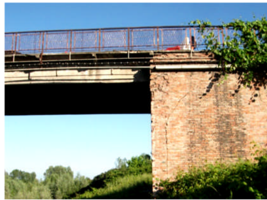
Figure 5.5 – Typical cracking in the brickwork bridge abutments of Bomporto Bridge.
