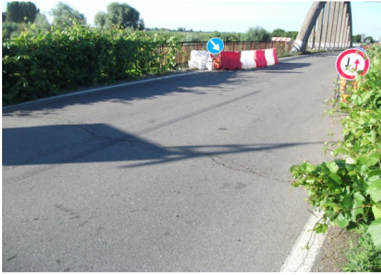
Figure 5.6 – Minor cracks in road surface due to damage to masonry abutments beneath.
