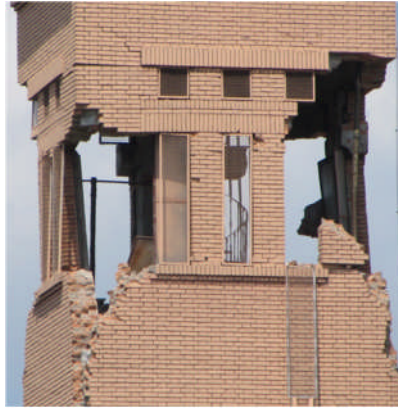
Figure 4.46 – Severely damaged tower in Concordia.
