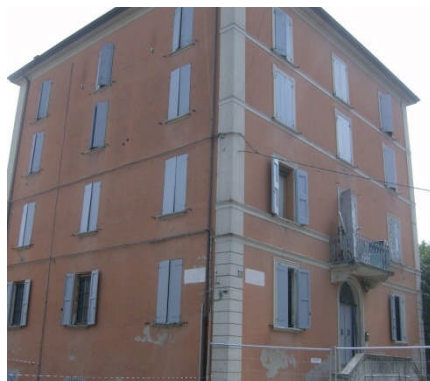
Figure 4.18: Typical quoins on both edges of the facades. The building on the corner between Via Guglielmo Marconi and Via Costa in Crevalcore has suffered shear failure in the spandrels.
