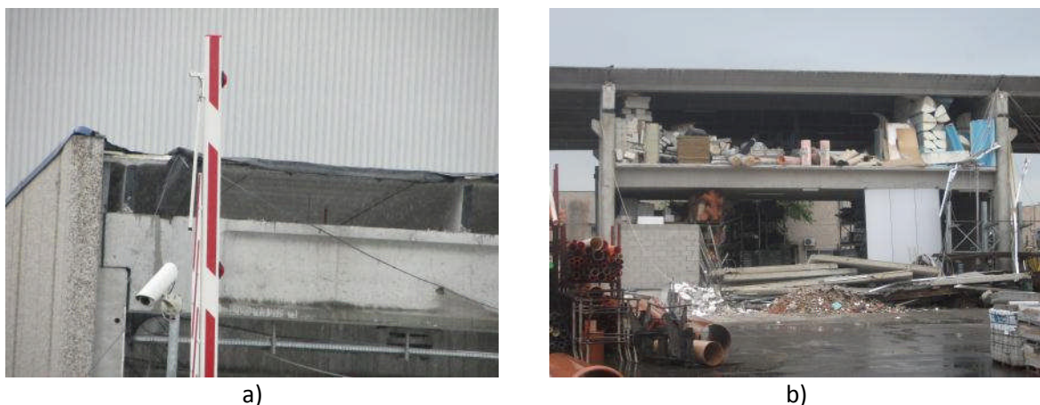
Figure 4.57 – a) Detail of a transverse double T-beams as a roofing system of a warehouse in San Giacomo Rancole b) Corrugated precast RC sections as roofing system for a warehouse in San Giacomo Rancole.
