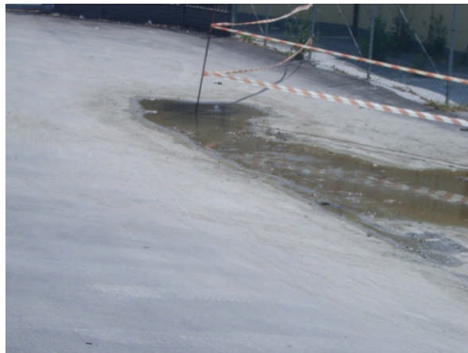
Figure 5.2 – Ponding of sewage at foul manhole in San Felice sul Panaro.
