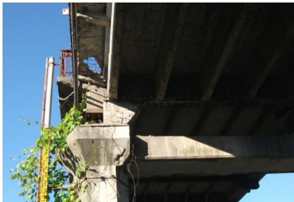
Figure 5.4 – Existing rusted rebar exposed prior to earthquake (Bomporto Bridge).
