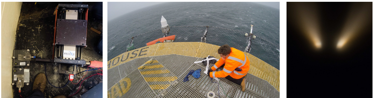
Fig. 6. Bishop Rock: Setting up shaker and accelerometers in battery room; weather protection for helideck sensors; twin beams in foggy night.
