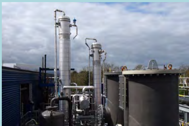
Biohydrogen plant in Swindon (UK)
