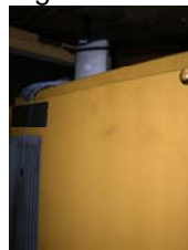
Figure 4 – Compressor Hot Air Exhaust
