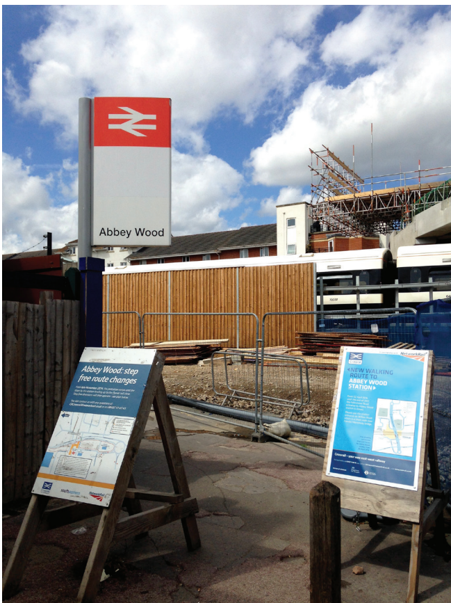
Figure 4.11. Construction at Abbey Wood station in preparation for the arrival of Crossrail. Source: Author (2016).
