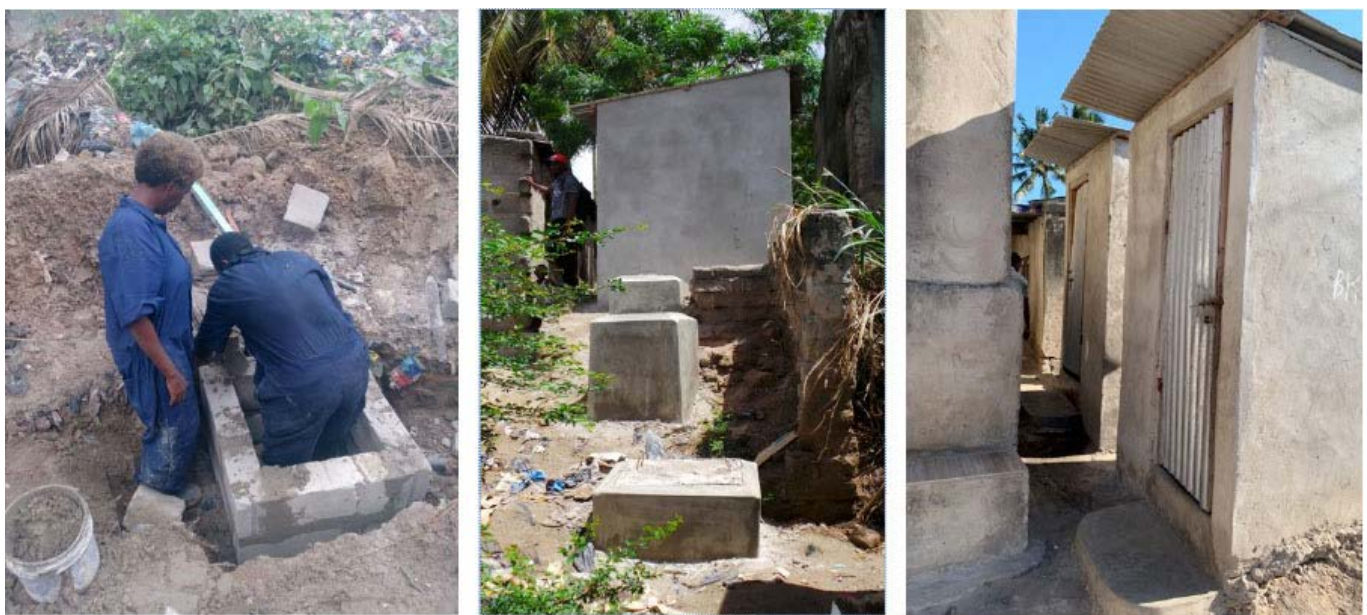
Figure 3 Inspection chambers along the sewer line and newly constructed toilets connected to the scheme (photos by CCI and P. Hofmann)
