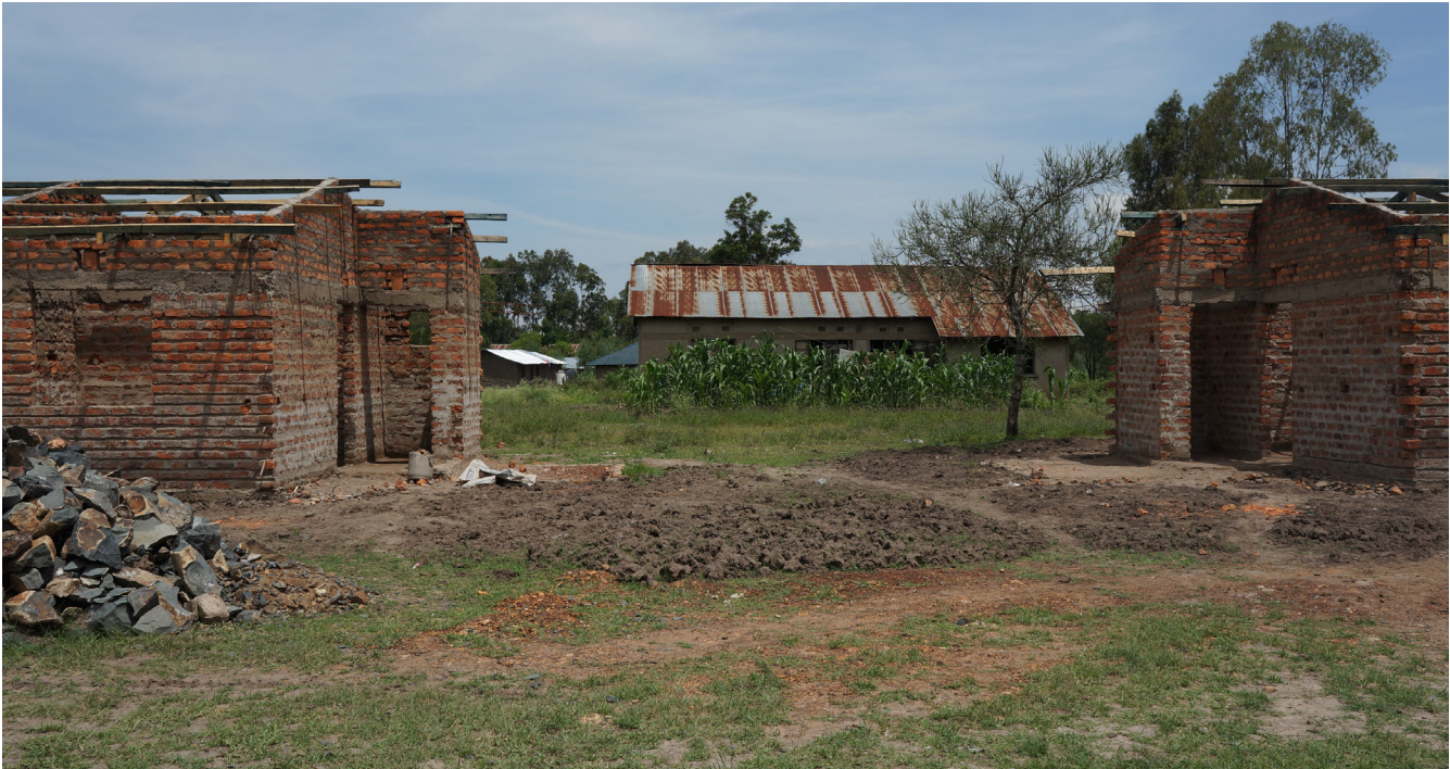
Picture 5. The first stage of construction at the Kibos project. Photo credit: Kai Mao.
