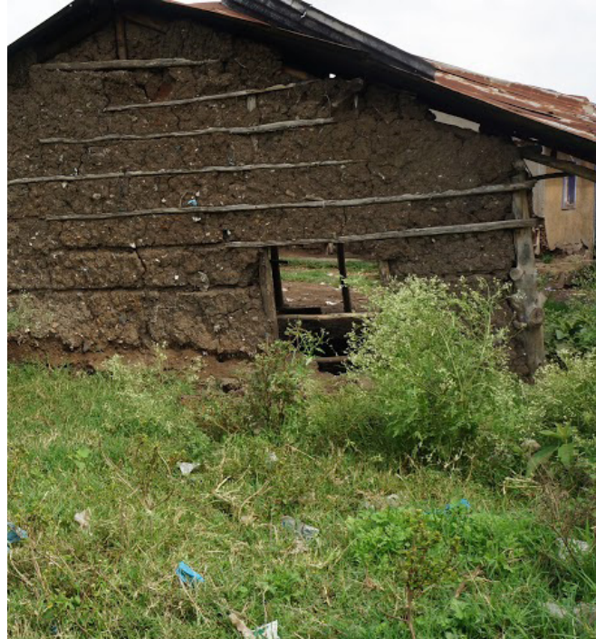
Picture 6. Traditional construction at risk of collapse. Photo credit: Kai Mao.
