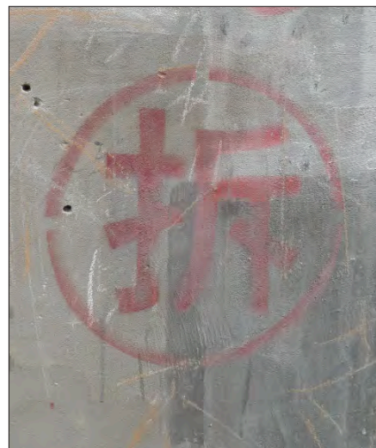
Picture 6: the dreaded symbol of a demolition order stamped on a building.
