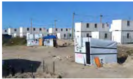
Above: Construction of new shelters at 'The Jungle', Calais. Photo by Giovanna Astolfo.
