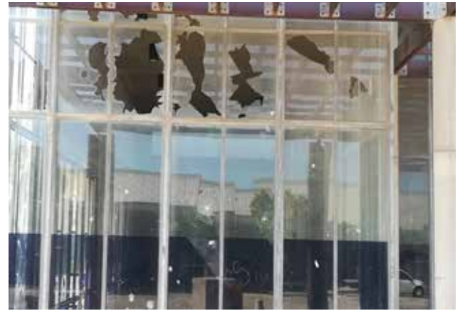
Figure 2: Damaged restaurant area, Red Location Museum (Zwai Mgijima, 2020).
