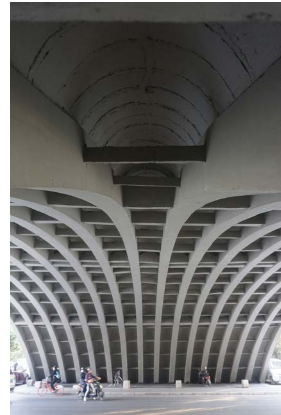
A view from beneath the double-curved part of the Yangtze River Bridge, Nanjing. (photographed by Yichuan Chen, 2020)
