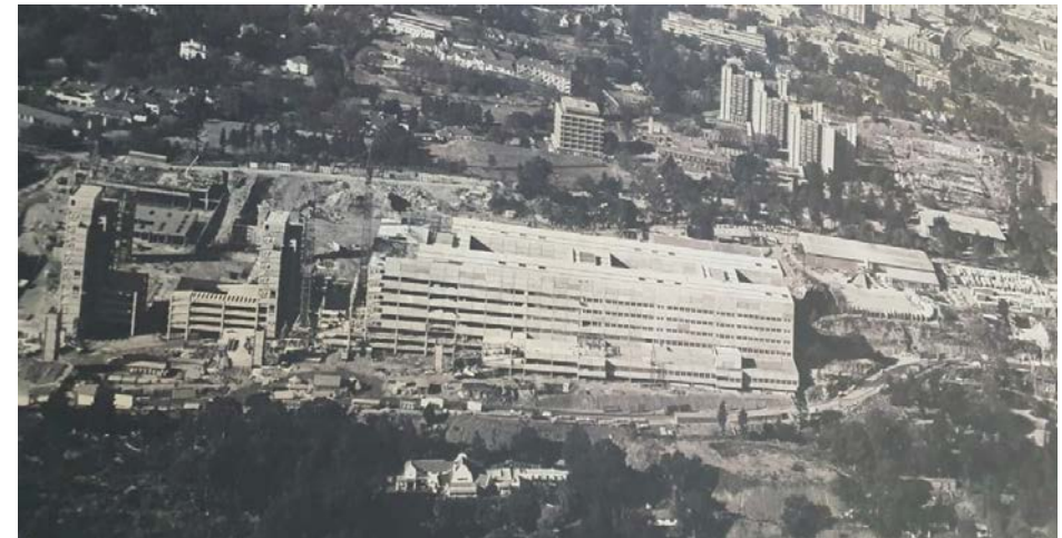
Johannesburg General Hospital under construction, c.1982. (Source: Building and Facilities Manager, Charlotte Maxeke Johannesburg Academic Hospital, July 2022)
