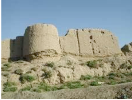
Part of the defensive circuit of Abdullah Khan Kala showing the wall, a guard tower (one of 48), moat and eroded defensive wall.
