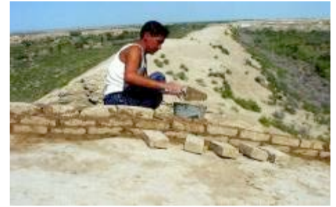
New wall built at the top of the defensive wall at Gyaur Kala redirects rainwater to stop erosion.
