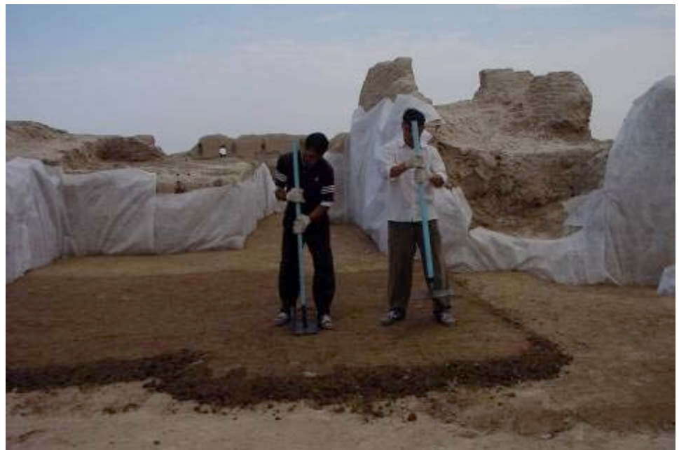
Tamping down backfill material in Shariyar Ark to conserve the archaeological remains. In the background is 'geo-textile' which covers the walls and allows them to 'breathe' through the backfill.
