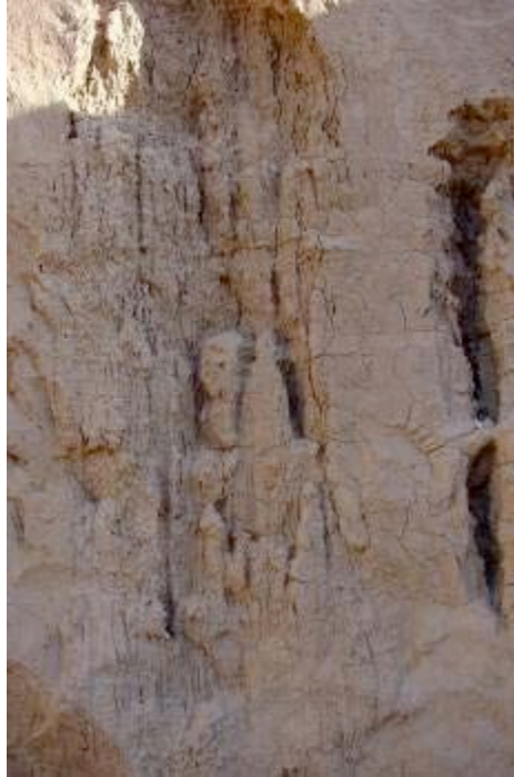
Rainwater runs down the face of part of a wall in Gyaur Kala creating gullies and damaging the structure.
