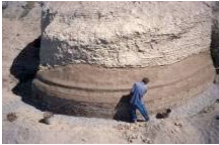
Repairing the base of one of the towers at Abdullah Khan Kala.
