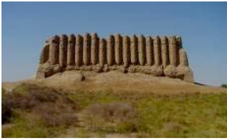
Damage at the base of the south wall of the Great Kyz Kala, with repairs at each end to stop the walls collapsing.
