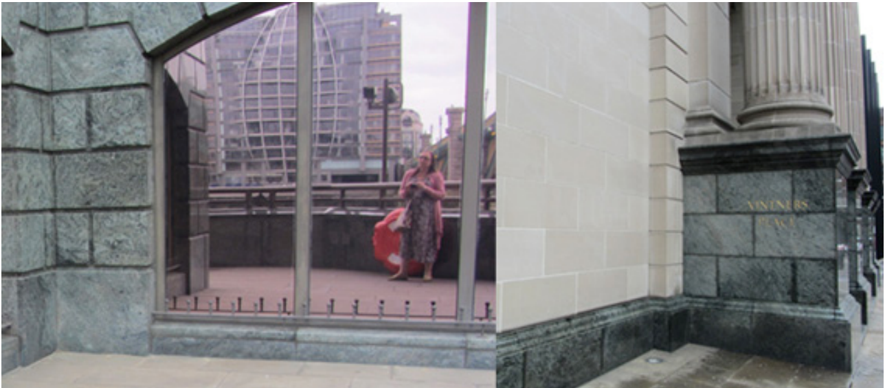
Vintner's Place: Left, Verde Candeias clads the foundation courses of the building. Right, Verde Candeias with Indiana Limestone above.
