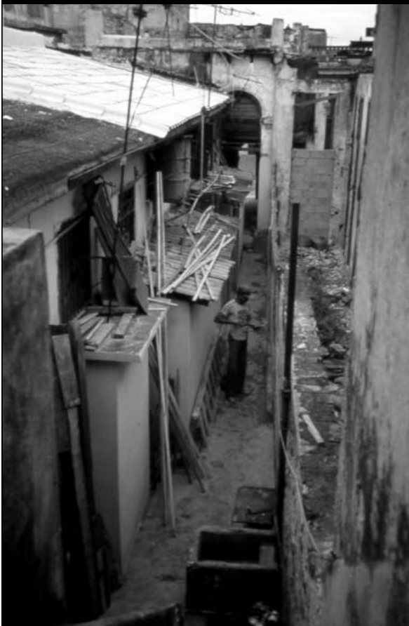
Photo 3. Atarés Tenements where Residents have Expanded their Units into the Narrow Courtyard. The Leaking Roof is being Repaired with Roof Tiles Produced on Site with Low-cost Technology
