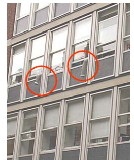
Figure 8 - Portable Units' Exhaust pipes
