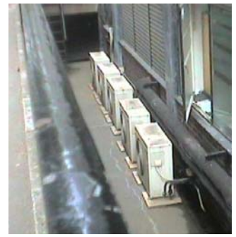
Figure 4 - Condensing units located below pavement level
