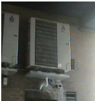
Figure 1 - Split AC system condensing units
