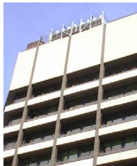
Figure 2 - Wet cooling tower
